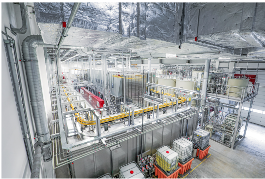
In 2020 Brose commissioned a zero-emission paint plant in Taicang/China.
